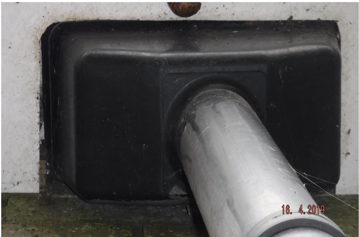
Photograph 7. Small gaps around a drain pipe on the north aspect of the building.
