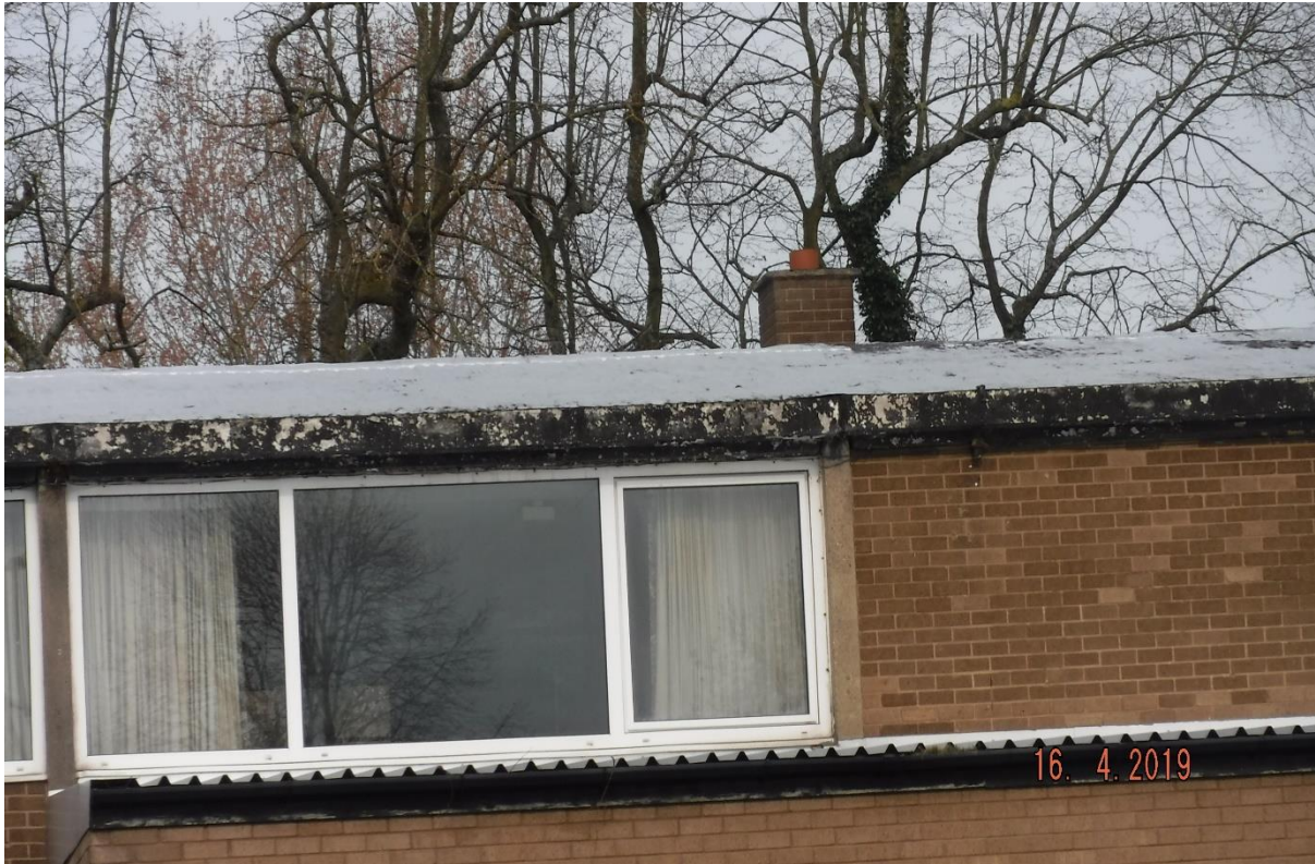
Photograph 5. Manmade material covering the pitched roof of the building. Corrugated metal covering the east flat roof section also seen below.
