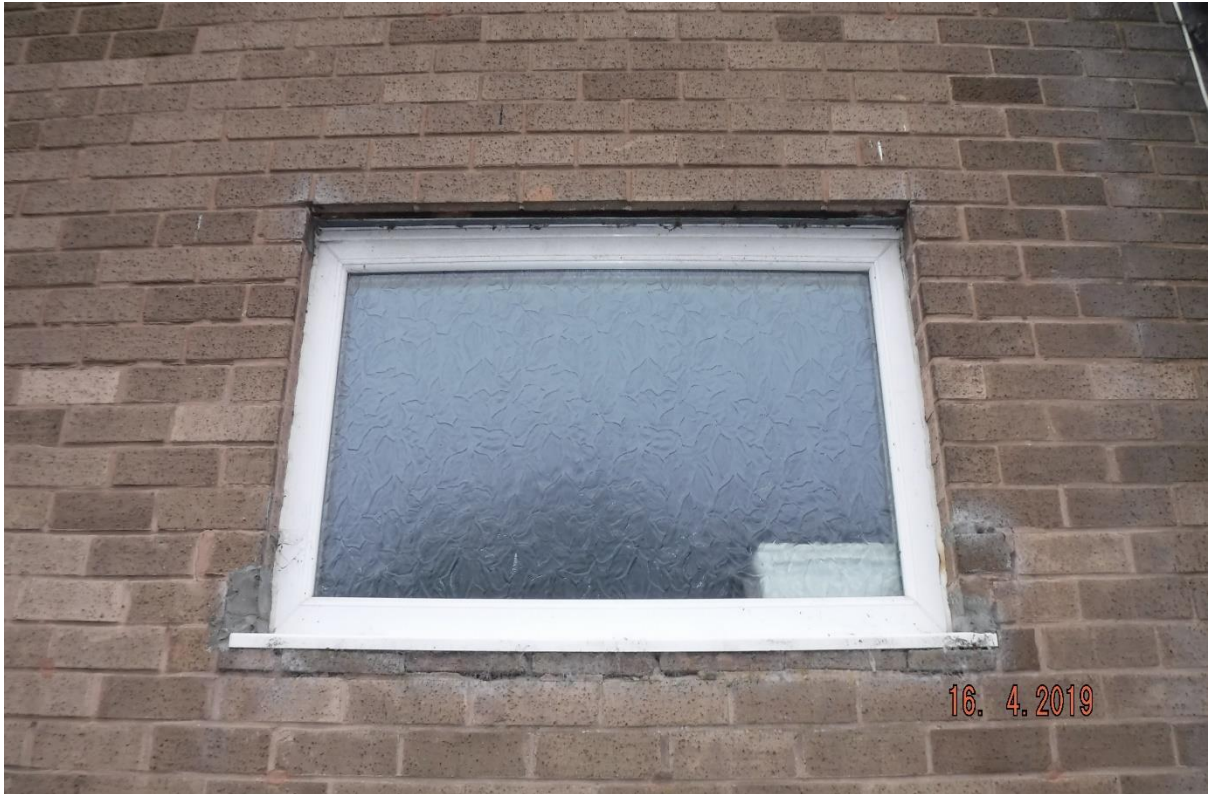
Photograph 8. The PVC windows and brickwork on the building are in good condition.
