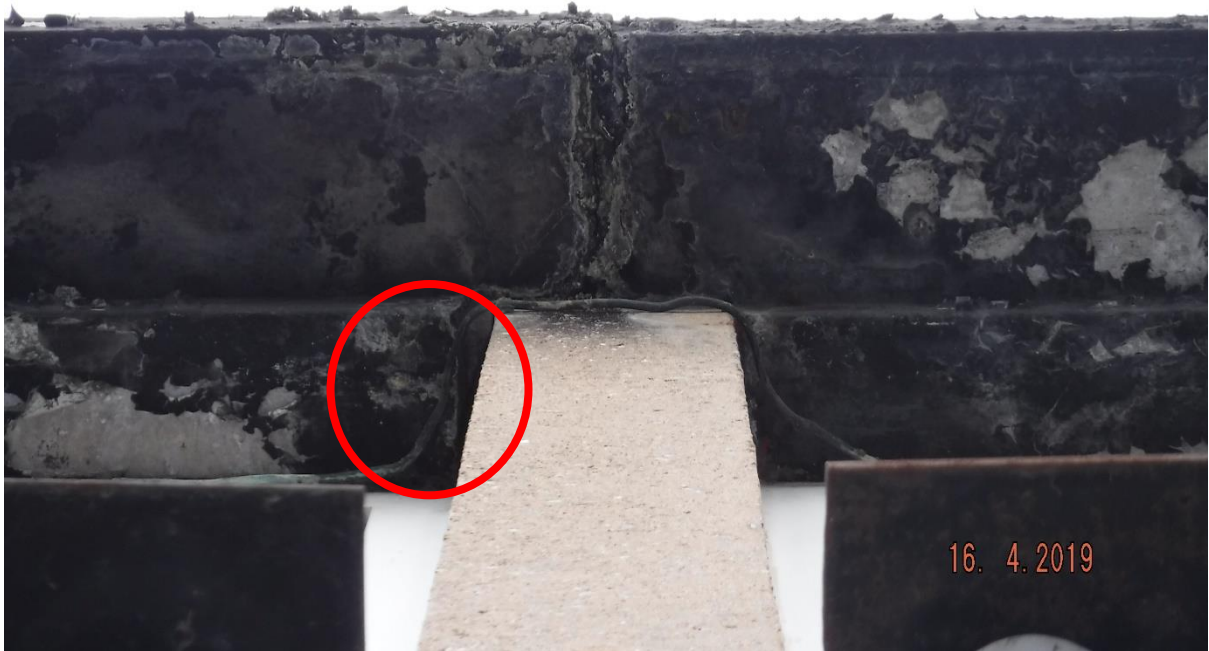
Photograph 6. Small gaps surrounding the concrete stanchions on the east side of the building.
